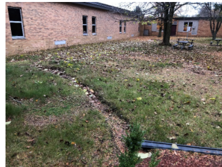
Lawn in poor condition. Swale cut for drainage.
