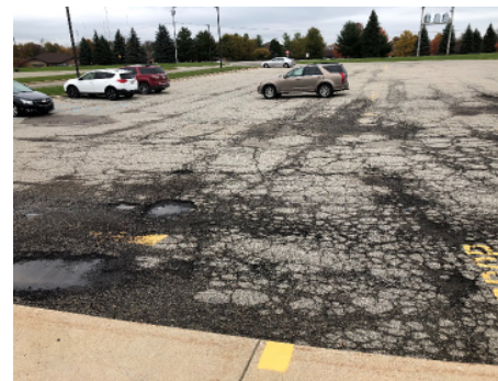
Parking lot asphalt in poor condition.
