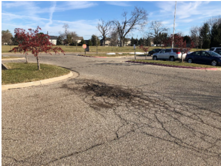
Asphalt beginning to show its age.
