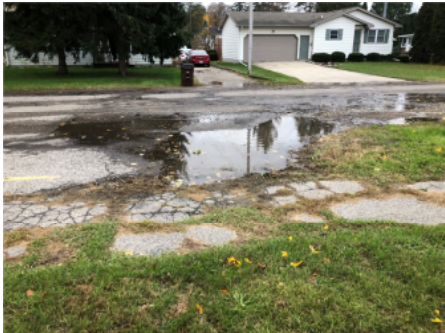
Public roadway/bus drop off area is in poor condition with standing water.
