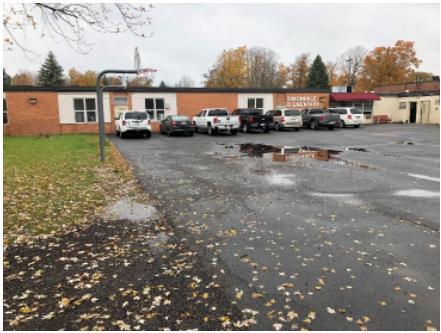
Courtyard does not have sufficient slope creating standing water within both pavement and greenbelt areas.
