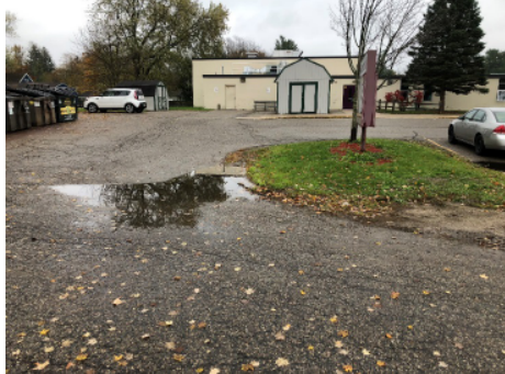
Water is trapped in low spots near edge of pavement accelerating pavement deterioration.
