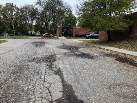
Parking lot asphalt in overall poor condition.
