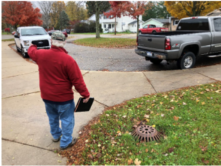
Storm water is not routed through the detention pond.
