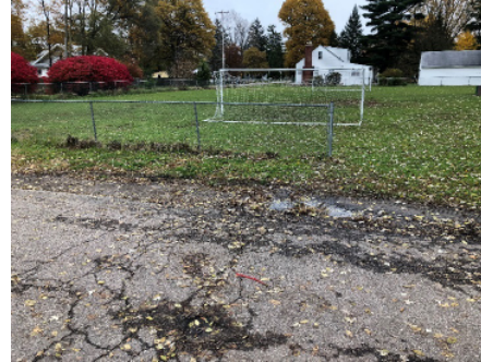
Areas of soil erosion.
