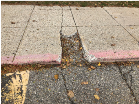
Sidewalk failing creating trip hazard.
