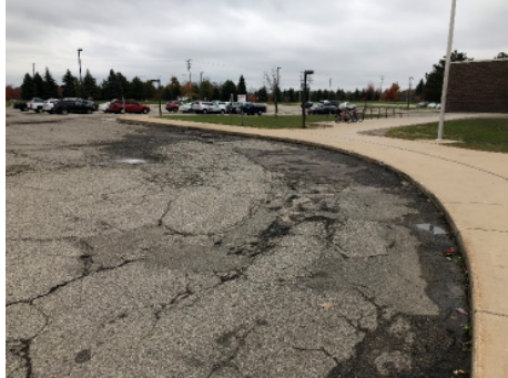
Parking lot asphalt in poor condition.
