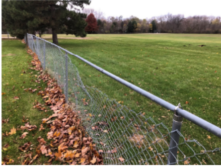
Fence in poor condition.
