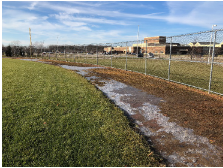
Minor drainage issues at softball field.
