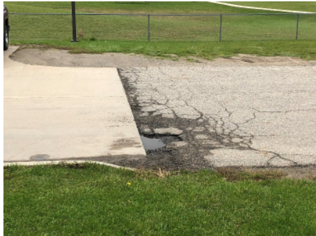
Water is trapped in low spots near edge of pavement accelerating pavement deterioration.
