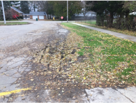
Perimeter of parking lot lacks curb and gutter with evidence of traffic rutting.
