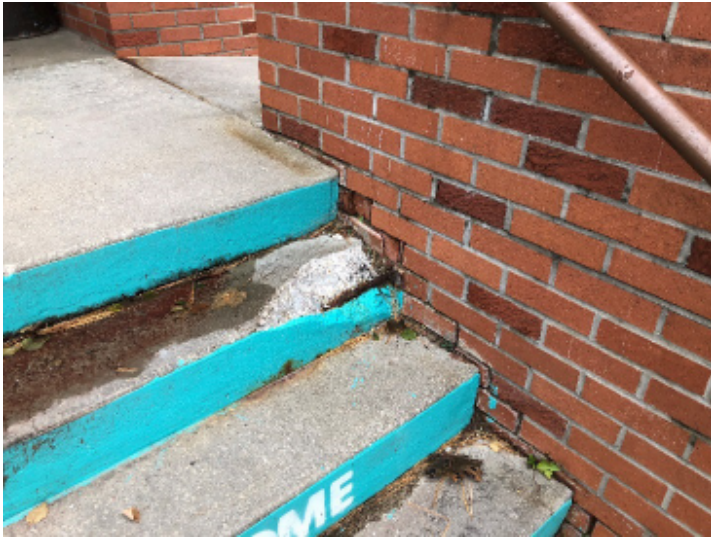
Steps failing with exposed rebar.
