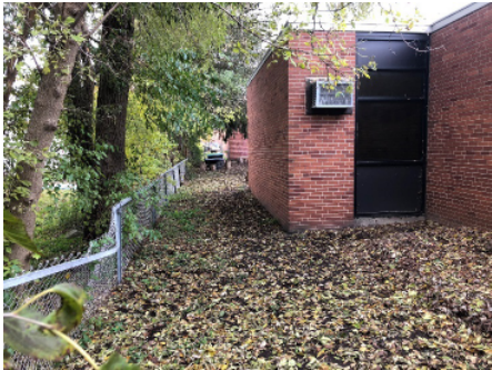
Fence is in poor condition.
