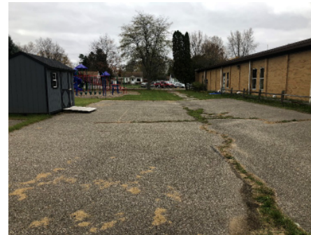
Asphalt in poor condition.
