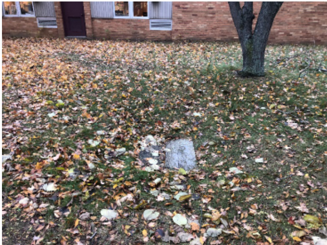
Manhole covered with plywood.
