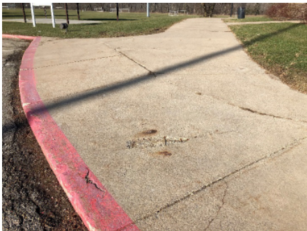
Sidewalk failing creating trip hazard.
