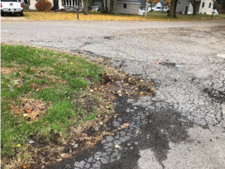
Water is trapped in low spots near edge of pavement accelerating pavement deterioration.
