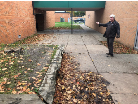
Landscaping upgrades are overdue.
