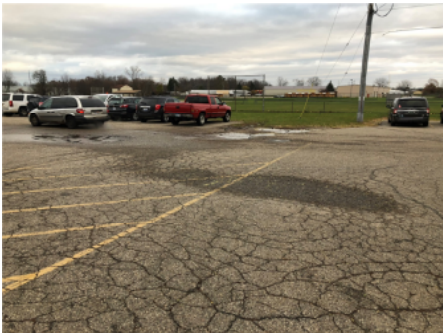
Parking lot asphalt in overall poor condition.
