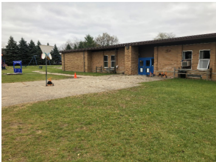
Asphalt play area in poor condition.
