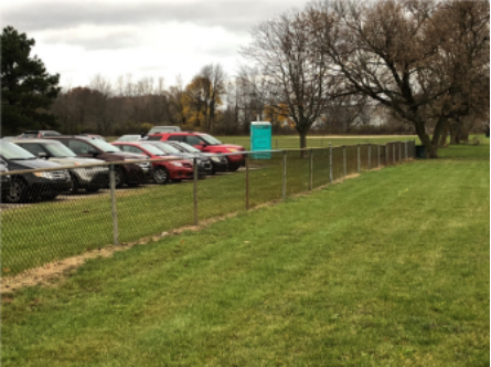
Perimeter fence is rusted and aged.
