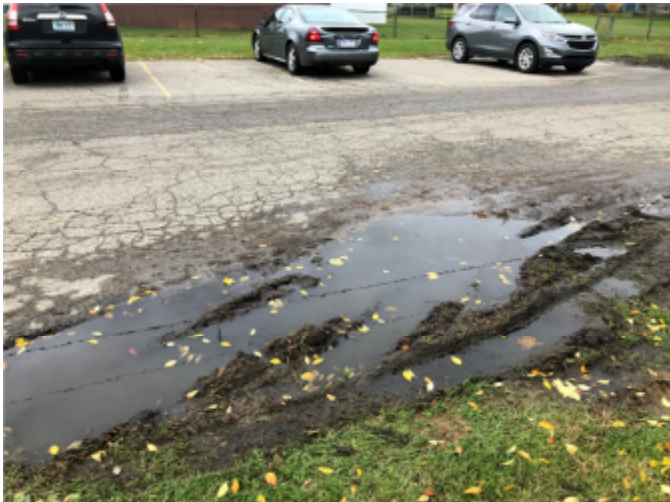
Pots holes and standing water.
