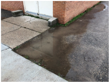
Asphalt is installed between building and playground. Slope tips towards building causing ponding water.
