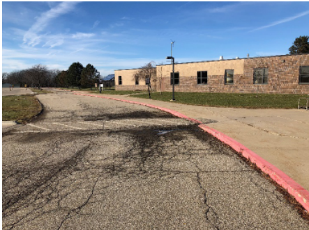
Bus loop road in poor condition.
