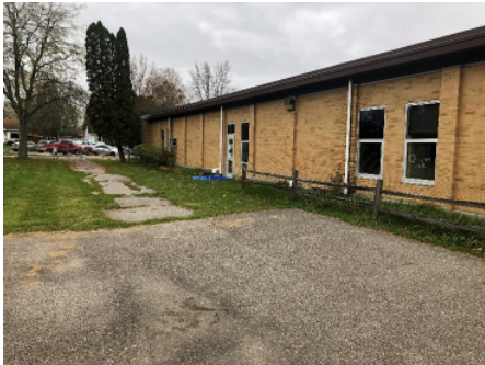
Asphalt pathway in poor condition.
