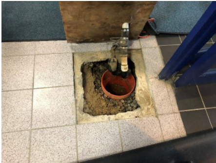
Makeshift sump pump in front entrance.
