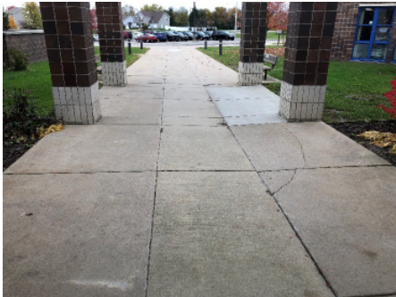
Swale in front walk is a result of storm sewer trench settlement.
