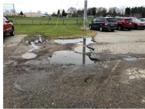
Pot holes and standing water.
