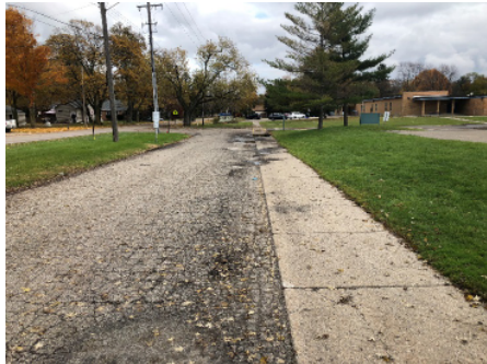
Bus loop asphalt and concrete sidewalk in poor condition.
