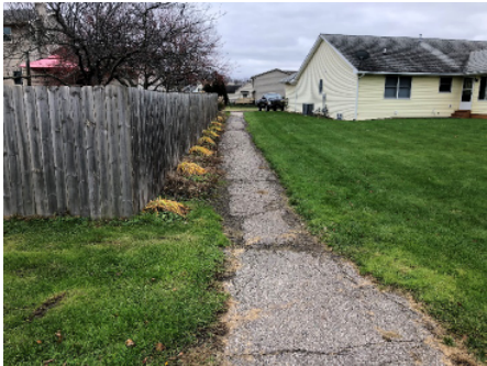
Pathway in poor condition.
