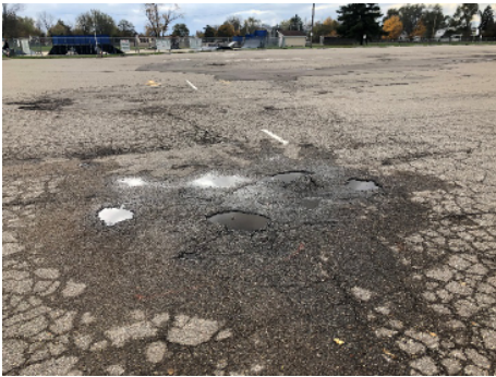
Parking lot asphalt in poor condition.
