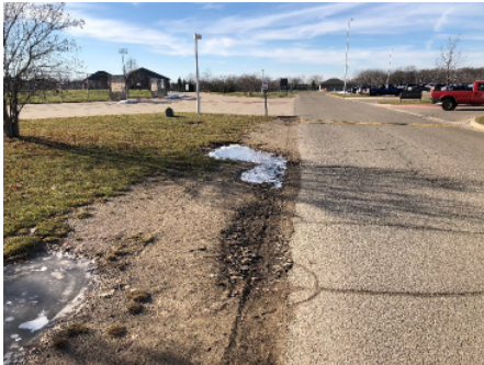
Consider addition of curb and gutter to protect asphalt.
