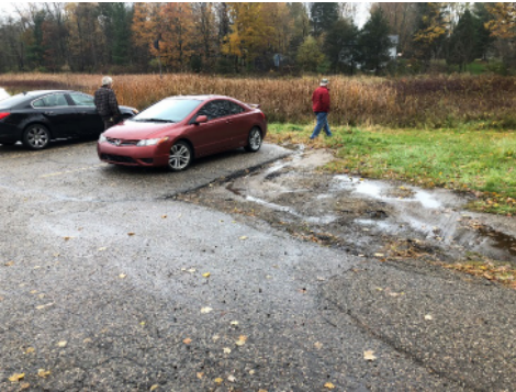
Landscape islands and perimeter of parking lot lack curb and gutter with evidence of traffic rutting.
