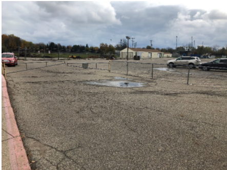
Standing water in parking lot. Additional storm sewer and/or parking lot regrading required.
