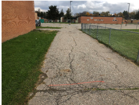
Asphalt drive/path in poor condition.
