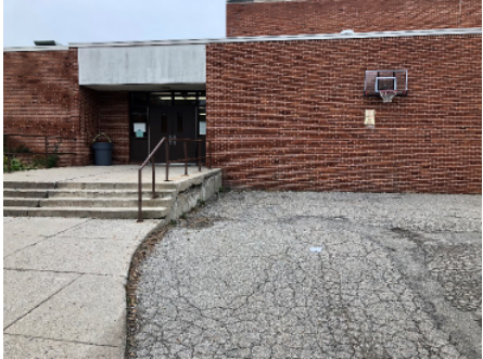
Courtyard asphalt and concrete stairs in poor condition.
