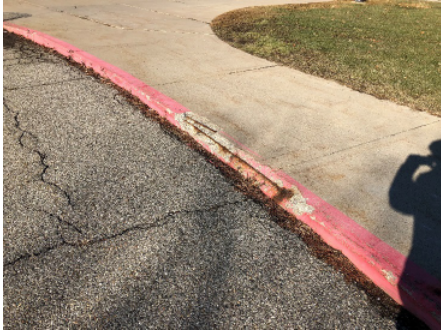
Standing water in parking lot. Additional storm sewer and/or loop road regrading required.
