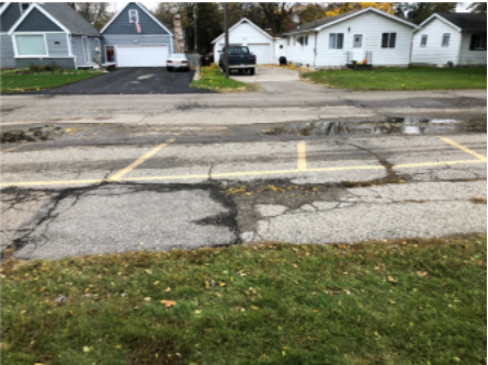
Public roadway/bus drop off area is in poor condition with standing water.
