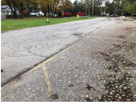
Public roadway/school parking in poor condition.
