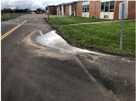
Standing water on new pavement. Additional storm sewer required.
