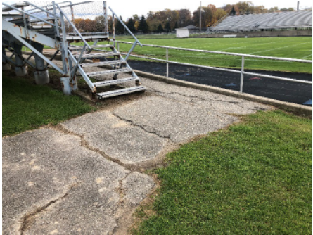
Pathway asphalt in poor condition.
